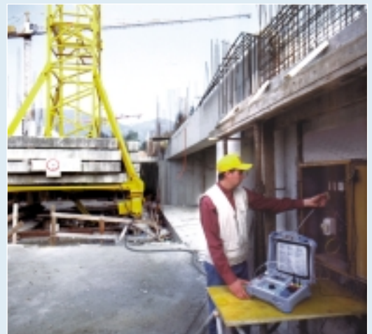
Testing of safety in a construction site on a switchgear
